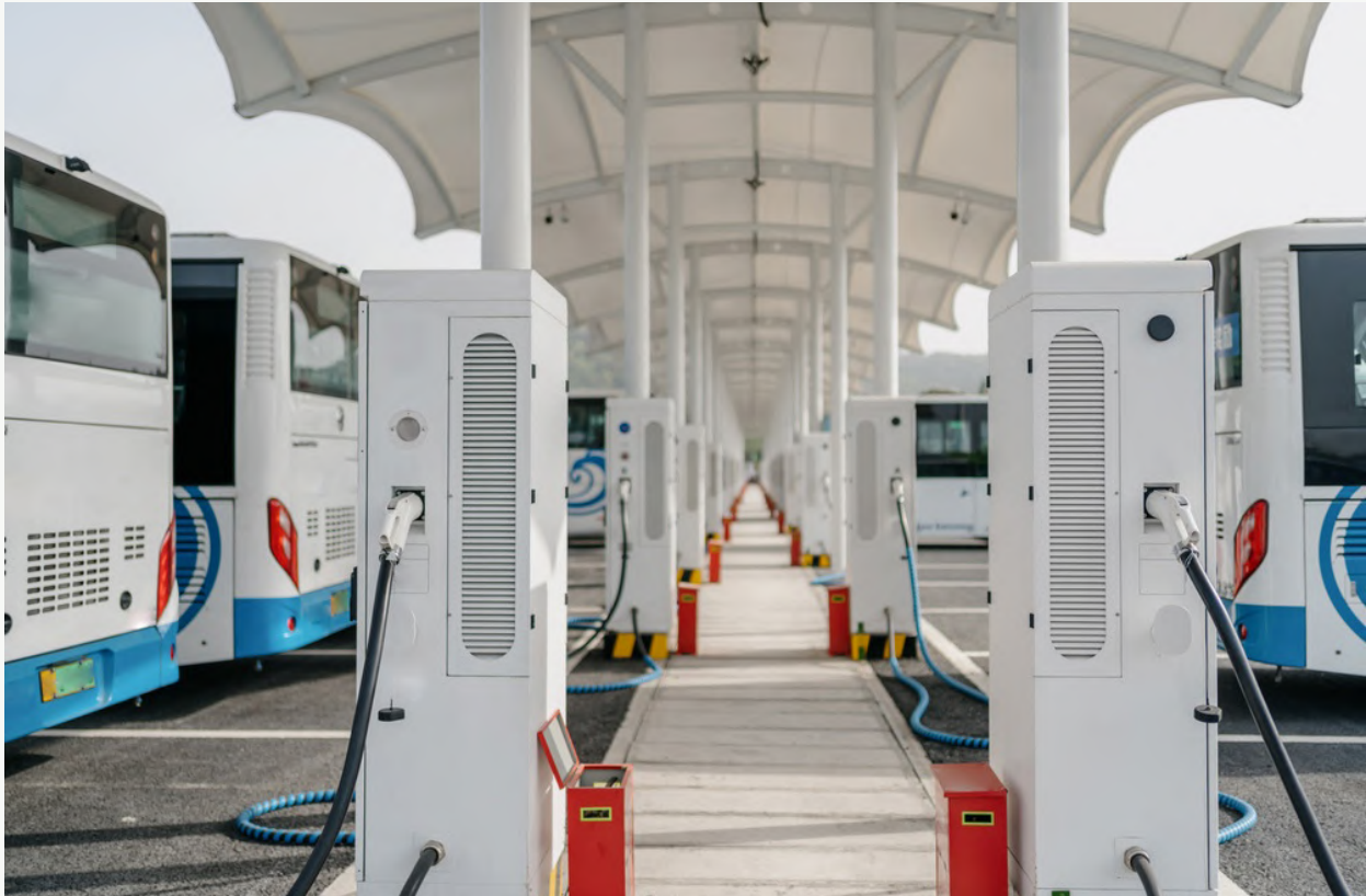
FIGURE 12: Dual Head Fast EV Charger Terminals
