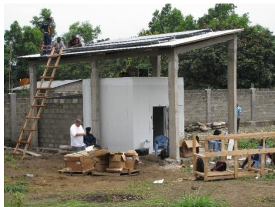
Figure 41. Insulated box with small commercial standalone solar installation above it
