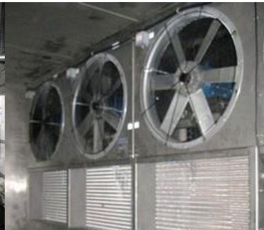
Figure 47. Example of high-volume freezer refrigeration equipment
