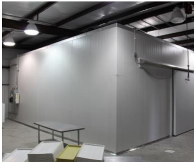
Figure 45. Example of a fish blast freezer
