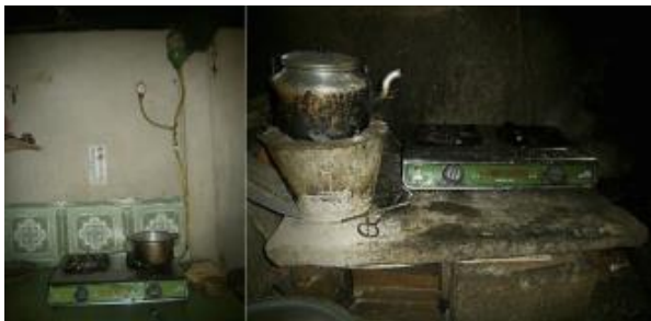
Biogas (Small-scale biogas plants in central Vietnam and biogas appliances with a focus on a flue gas analysis of biogas cookstoves (Roubik and Mazancova 2019))
