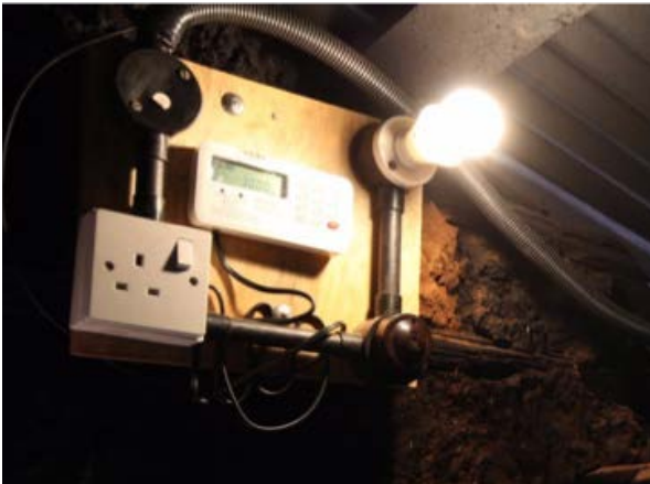
KPLC ready meter board
