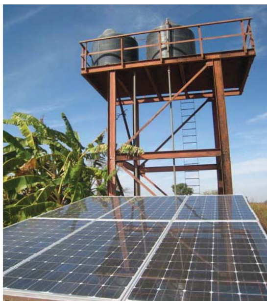
Figure 3.2: Solar Water Pumping System at Hospital at Bwiam, Foni Kansala District
